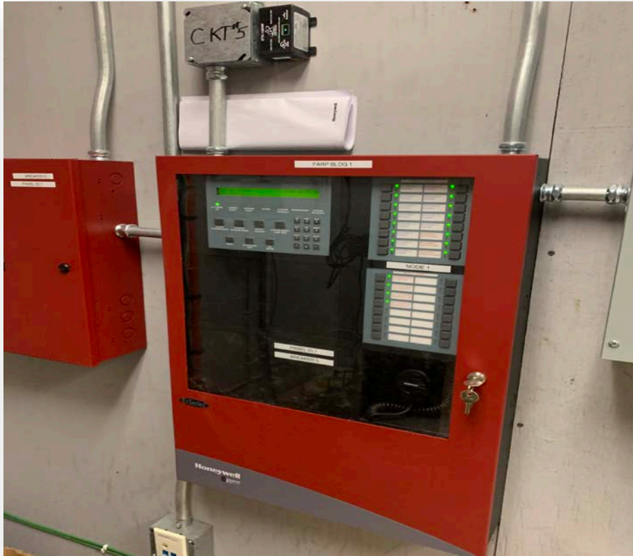
Fire Alarm System Replacement
